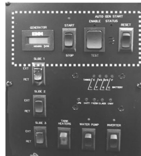
Command Center Panel
